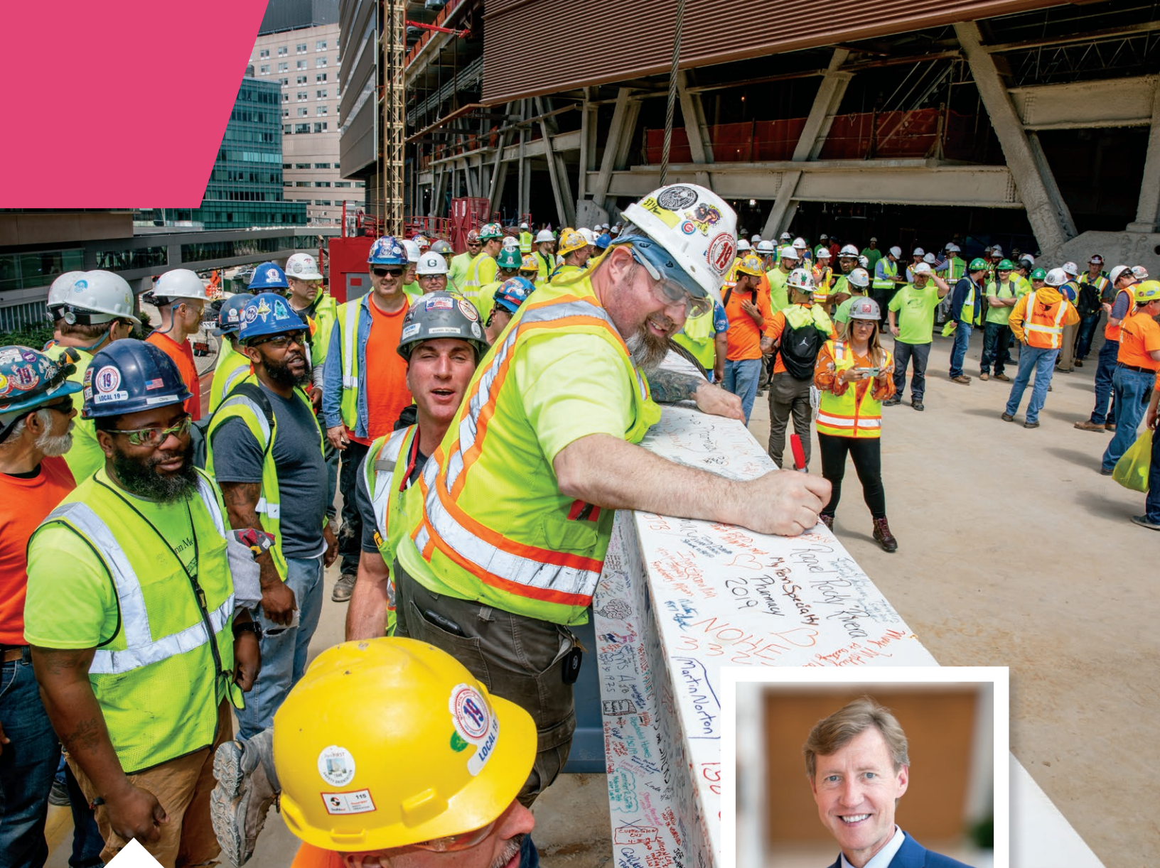
This May, crew members and supporters of Penn's Pavilion celebrated the traditional construction topping-off ceremony by signing the last beam before it was placed.
